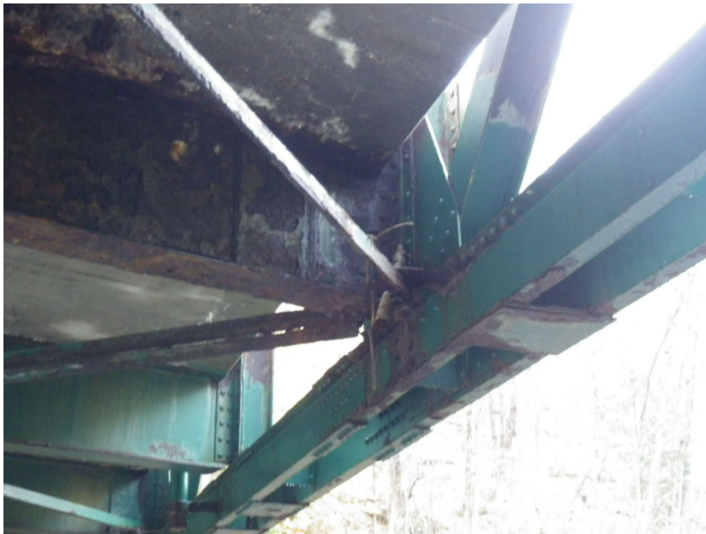
Picture 11: Deteriorated Floorbeam
