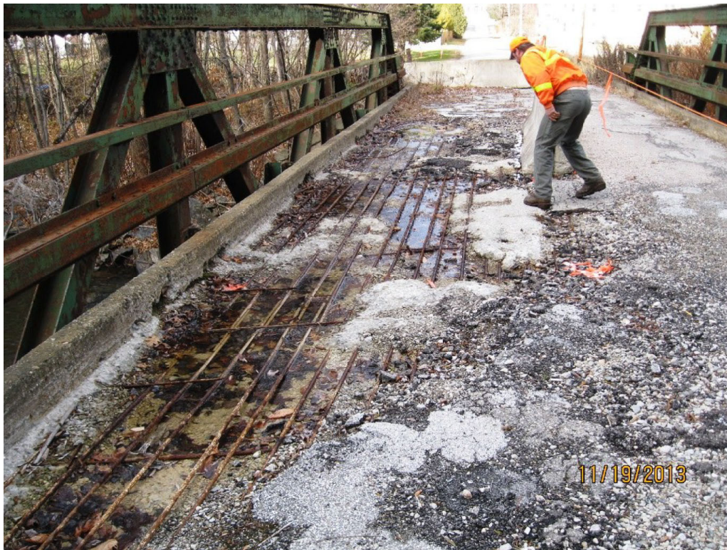
Picture 5: Exposed Reinforcing Steel on Deck
