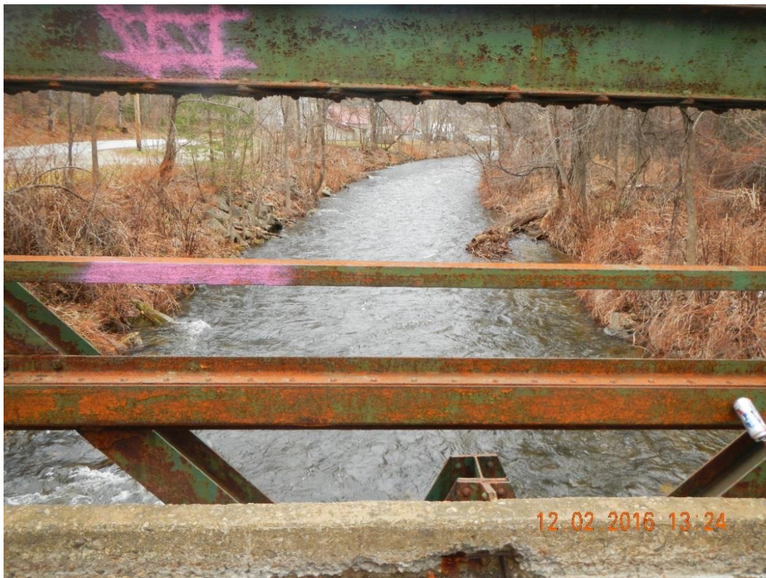
Figure 4: Cobbles and boulders visible on river banks on upstream side of bridge.
