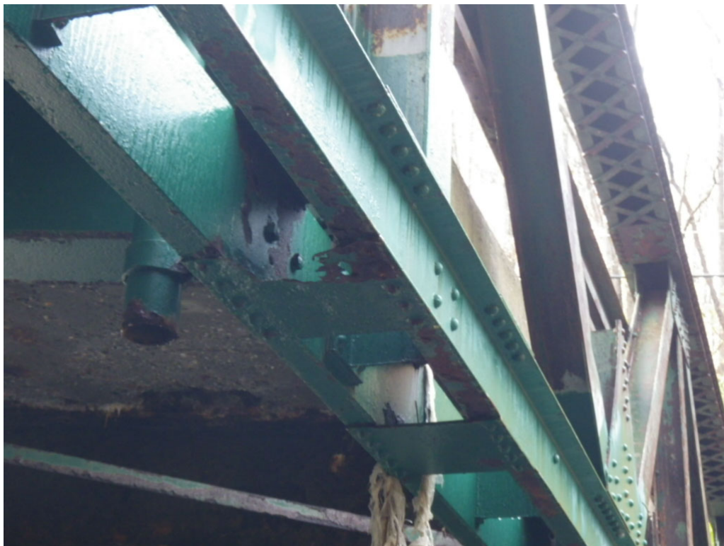
Picture 12: Section Loss at Gusset Plate
