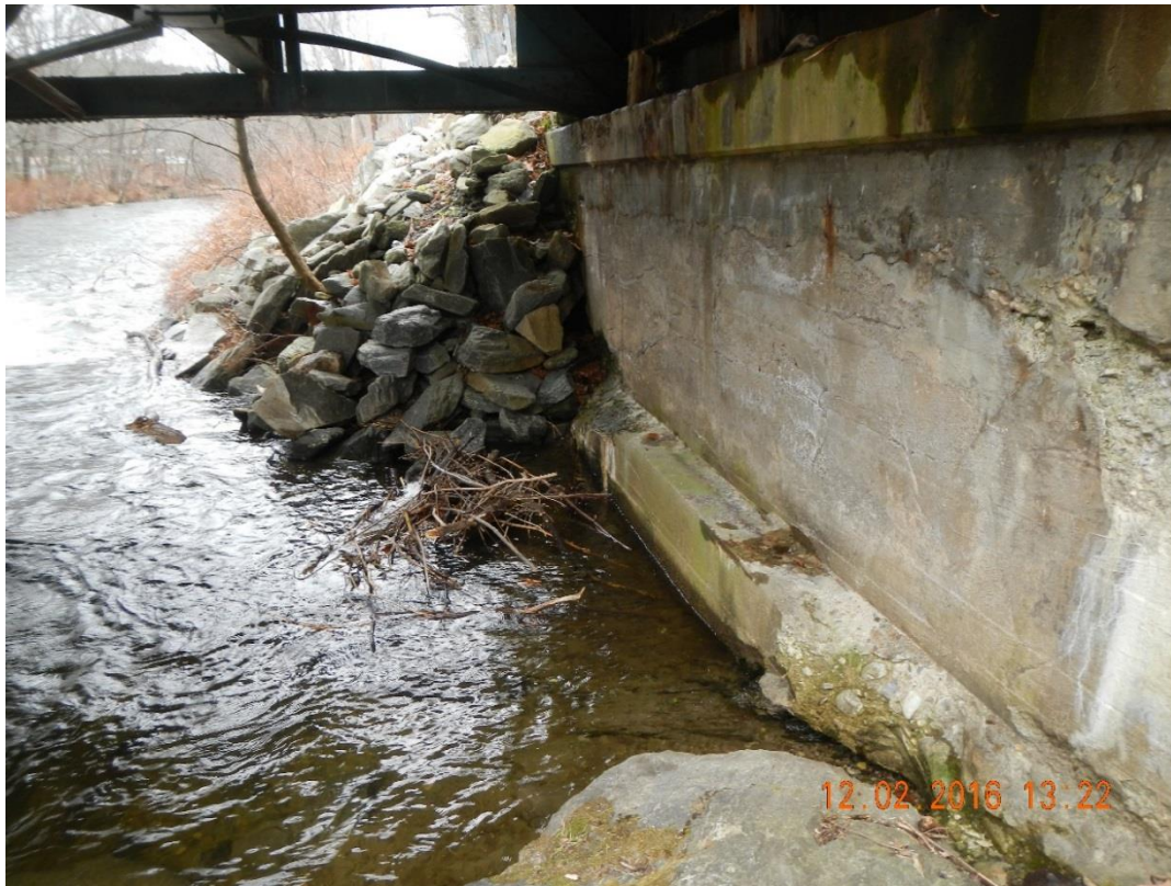
Figure 6: Southern abutment; note visible cracking and spalling of concrete.
