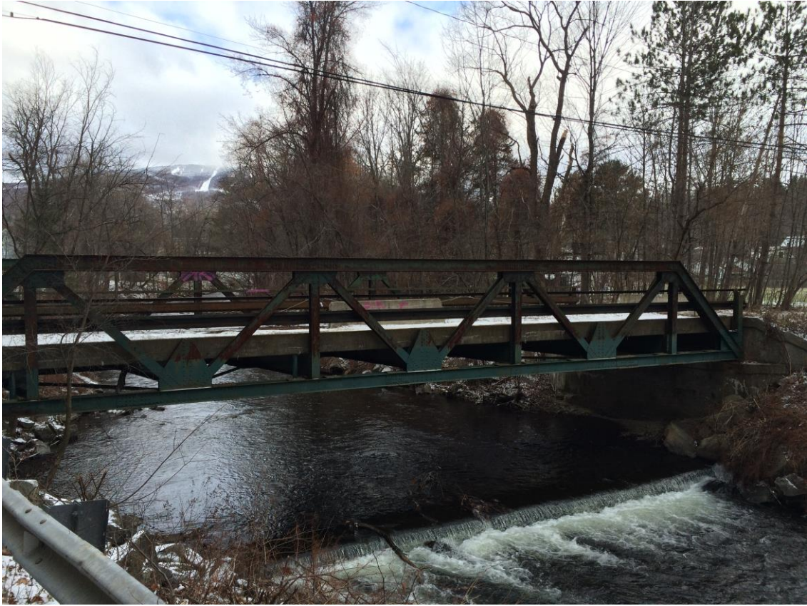
Figure 4. Bridge No. 57 with extant mill dam in foreground, looking west from Pleasant Street.
