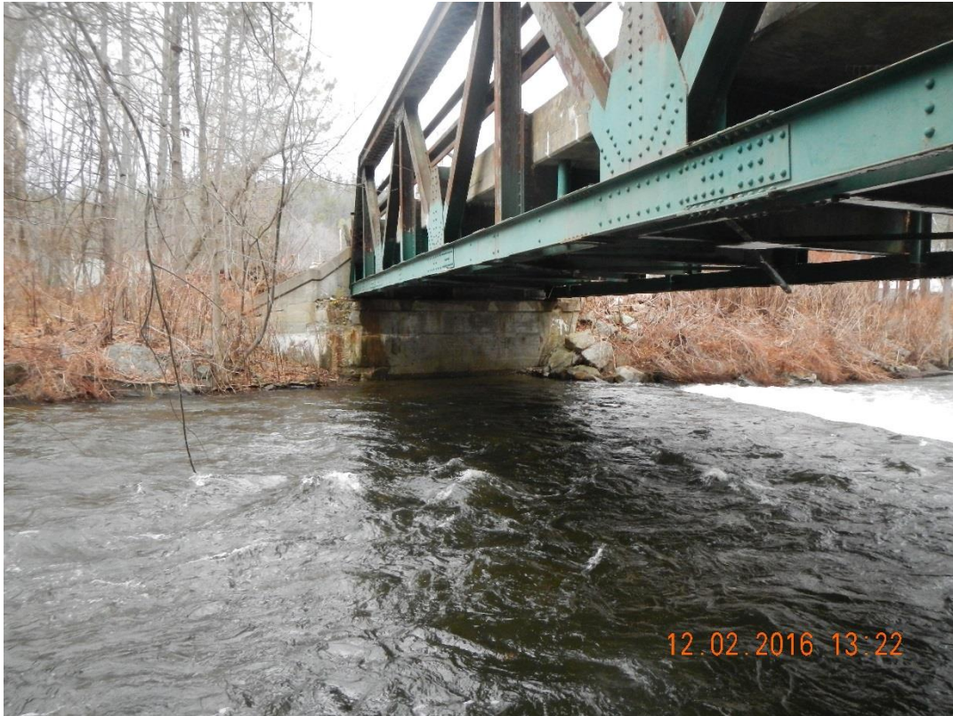
Figure 5: Northern abutment; note visible cracking and spalling of concrete.
