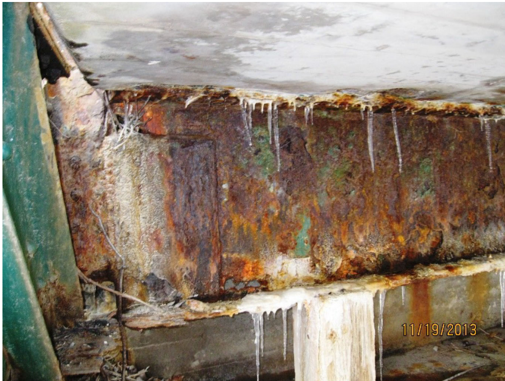
Picture 6: Deteriorated Floorbeam
